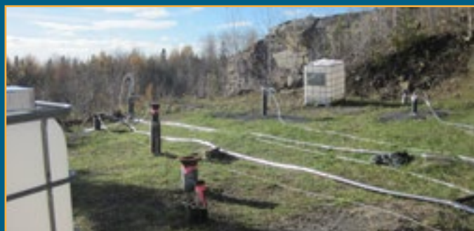
A bioremediation amendment recirculation system is being used at one of the TI waiver sites.
