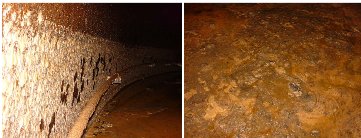
Figure 2-4. Corrosion in an AST storing a biodiesel blend: tank wall (left) and tank floor (right). Source: BP.
