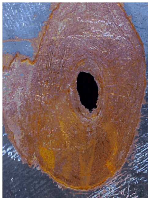
Figure 2-8. Corrosion in an E85 tank previously used to store E10. Source: Iowa Department of Natural Resources.
